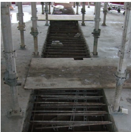
Pour Strips restrict site access, cause a trip hazard and delay progress on site
