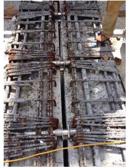
..... Installation of the specially modified Ancon DSD connectors for high shear load transfer.
